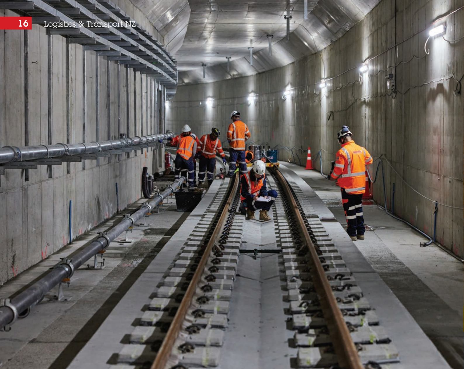
The beginning of the fit out of the tunnels as part of the City Rail Link project. Photos: City Rail Link
